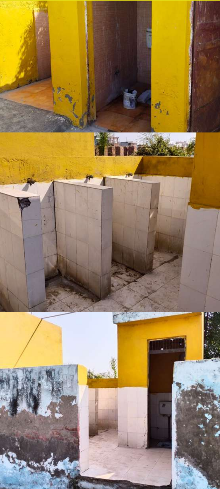
In Picture - Garhi Bohar Govt. school washrooms before our intervention
